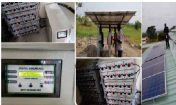
Fig. Photograph of 7.5 kWp remote microgrid with Solar PV- Battery –Diesel genset in Enable Project in Uganda
