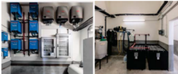
Fig. Photograph of 82 kWp grid-connected Microgrid with Solar PV- Battery –Diesel genset in Spain
